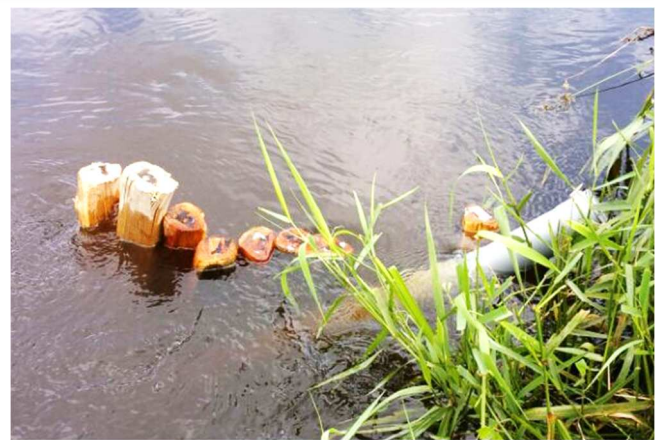
Fig. 2: Installation of an EXO1 multi-parameter probe in the pipe with protection against floating debris. Source: Lukas, LLUR
